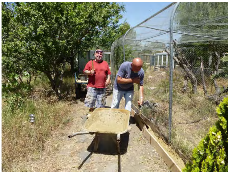
Terry having to threaten Chas with a hammer to make him help with concreting the fence base of an animal enclosure.
